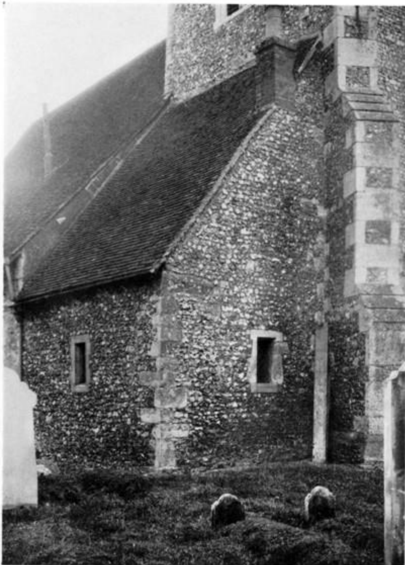
ANCHORAGE AT HARTLIP
